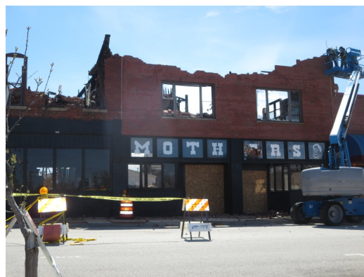
Extent of damage to Mother's Bar prior to being totally razed
